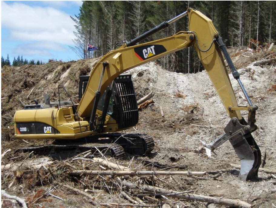
Figure 12. Excavator with a ripping and mounding head being used to prepare a site for planting.
